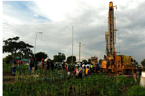
Using innovative rehabilitation and drilling technologies, MSF has drilled over 70 new boreholes in Zimbabwe. Photo: Samuel Sieber/MSF
