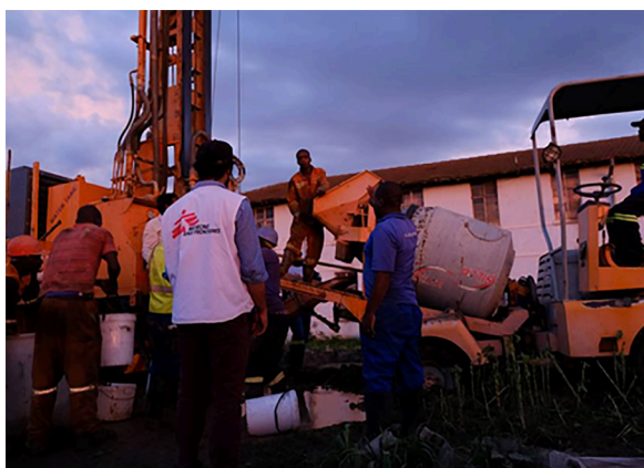
Cementation of the sanitary seal at the drill site in Mbare, Harare. Photo: Samuel Sieber
